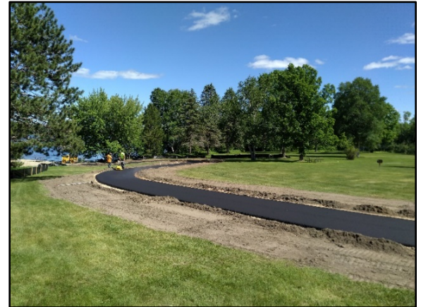
Paved pathway to lake at Gunn Park.
