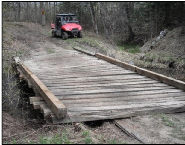
Balsam Creek snowmobile bridge in need of replacement.
